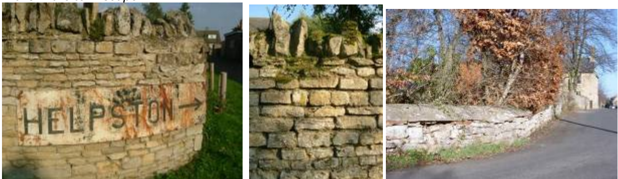
Wall in poor repair
